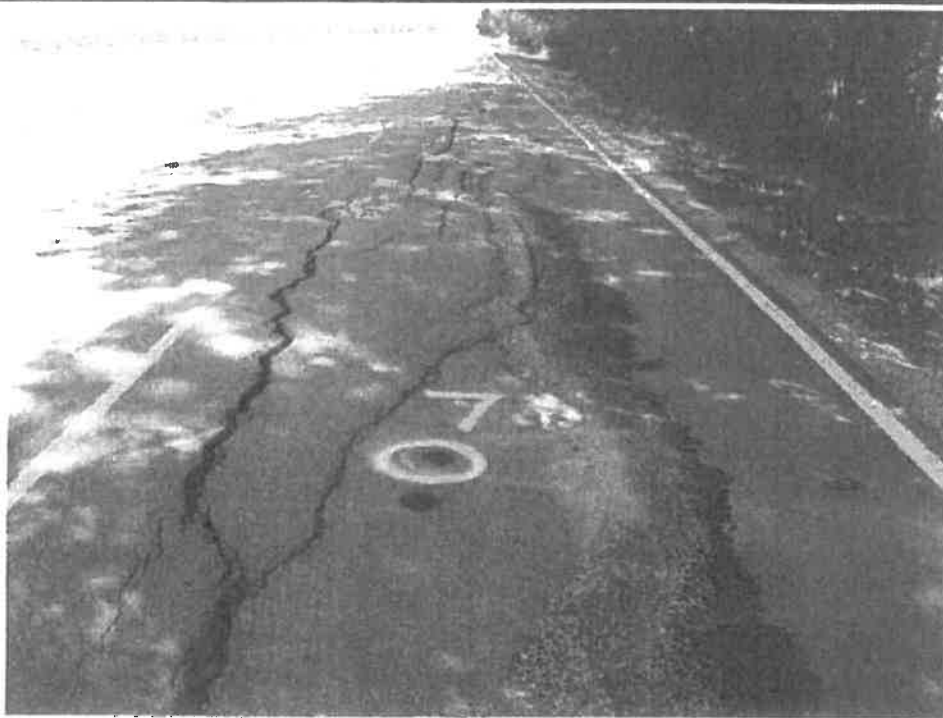
Photograph No. 9 – High severity cracking and previous maintenance near B7. Significant vegetation adjacent to east side of roadway.
