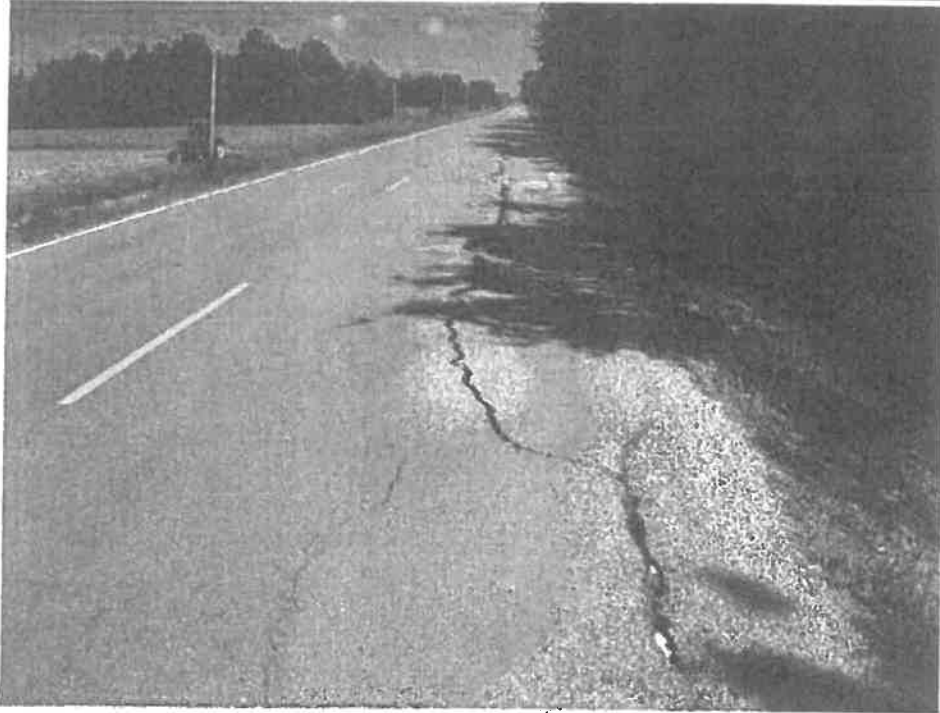
Photograph No. 3 – High severity cracking and differential movement near B2. Distresses located in northbound lane.
