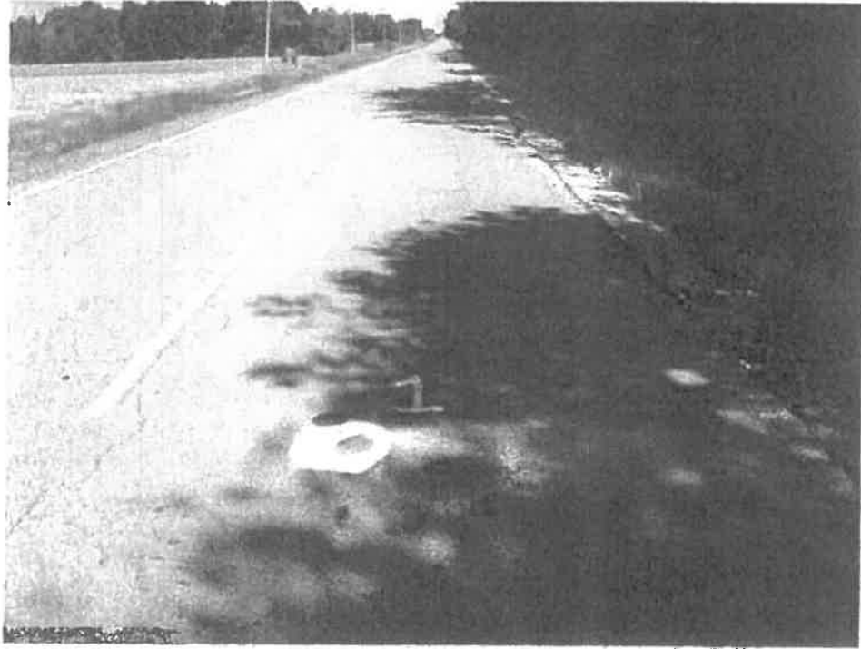
Photograph No. 1 – Typical pavement conditions near B1. Distresses located along east pavement edge.
