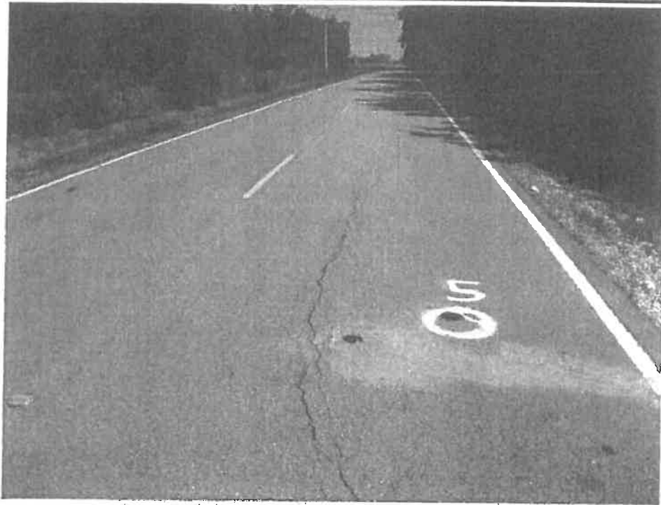
Photograph No. 7 – Low severity cracking near B5. Distresses located in northbound lane.
