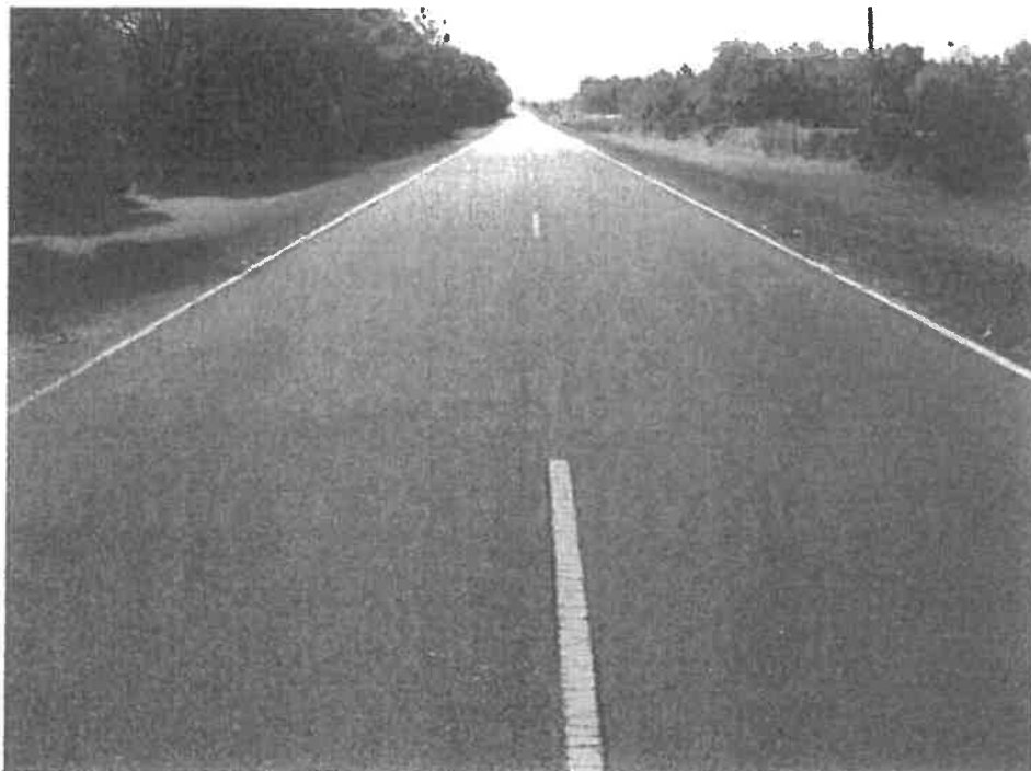
Photograph No. 6 – Fair pavement conditions. Shorter embankment with minimal vegetation adjacent to roadway.
