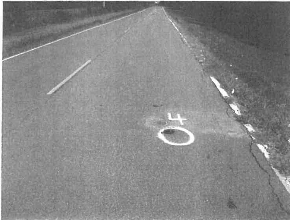
Photograph No. 5 – Fair pavement near B4. Low severity cracking along east pavement edge.
