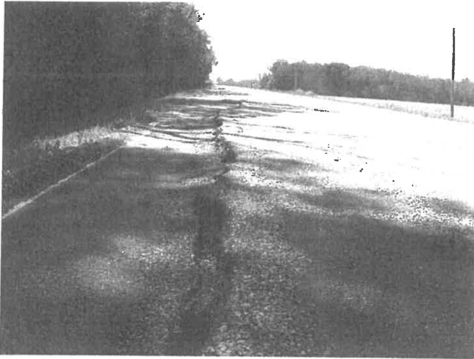
Photograph No. 4 – Close up of high severity crack and differential movement near B3. Distresses located along east pavement edge.
